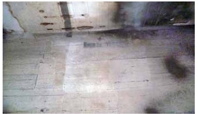
In one high level room there is evidence that it was once divided into levels. Photo Eva Westphal
